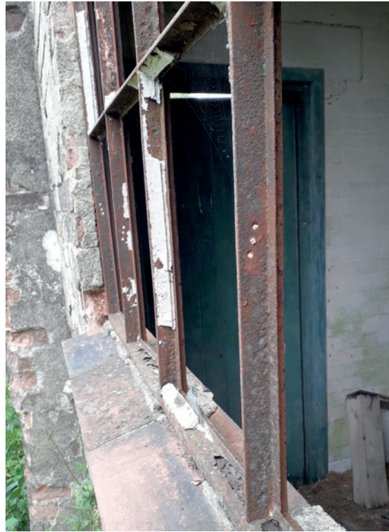
Distortion and loss where there has been water ponding
