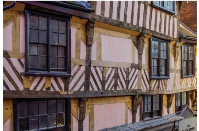
Early 17th century timber framed building in Wakefield, jettied after repair works in 2023
