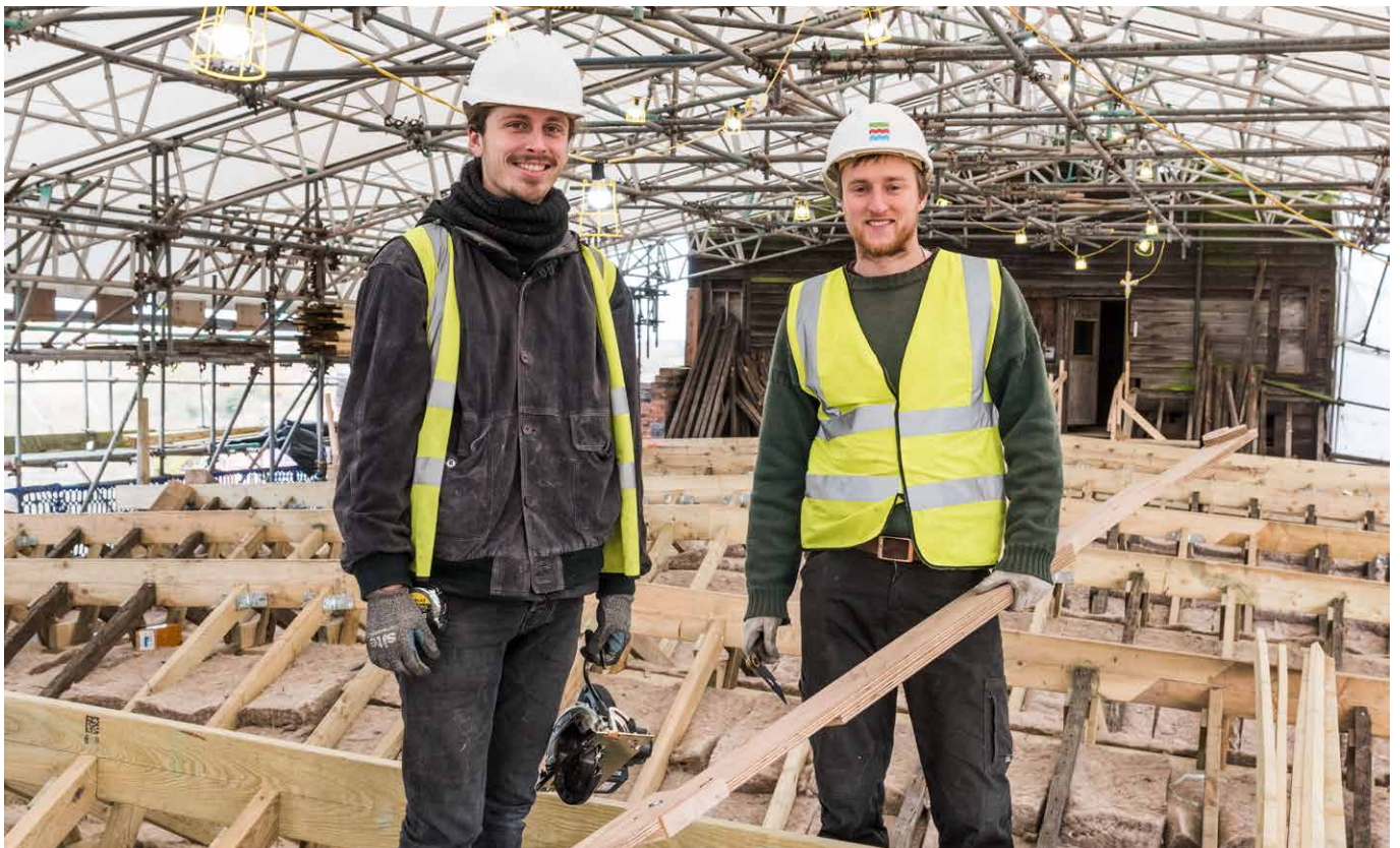
Prince's Foundation trainees learn new skills on the roof of the Main Mill, Shrewsbury Flaxmill Maltings, Shrewsbury, Shropshire. © Historic England Archive
