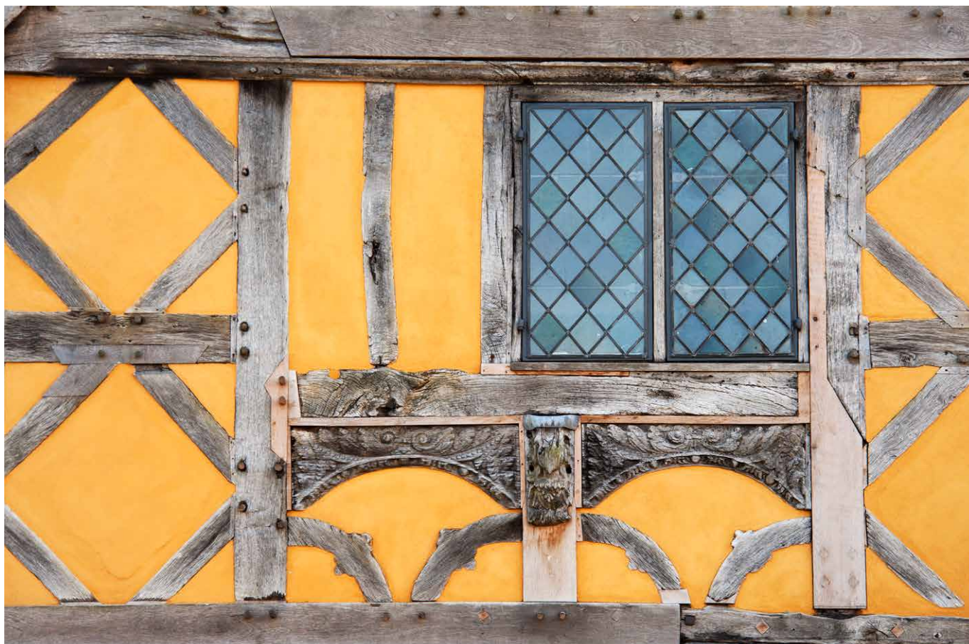
Detail of timber repairs from Gatehouse, Stokesay Castle, Stokesay, Shropshire. © Historic England
