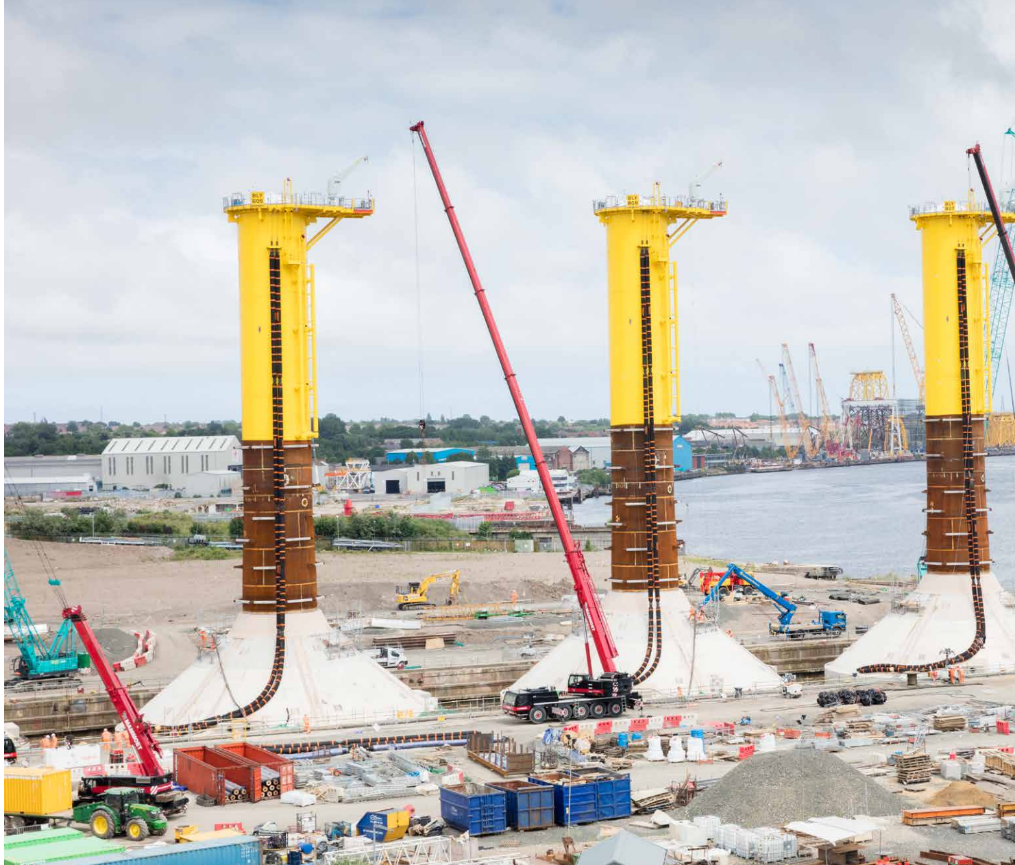
Blyth Offshore wind farm gravity based foundations under construction in 2017. © Historic England Archive
