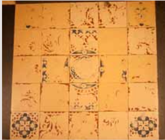
A badly worn section of encaustic tiles in St Stephen's Hall floor before conservation
