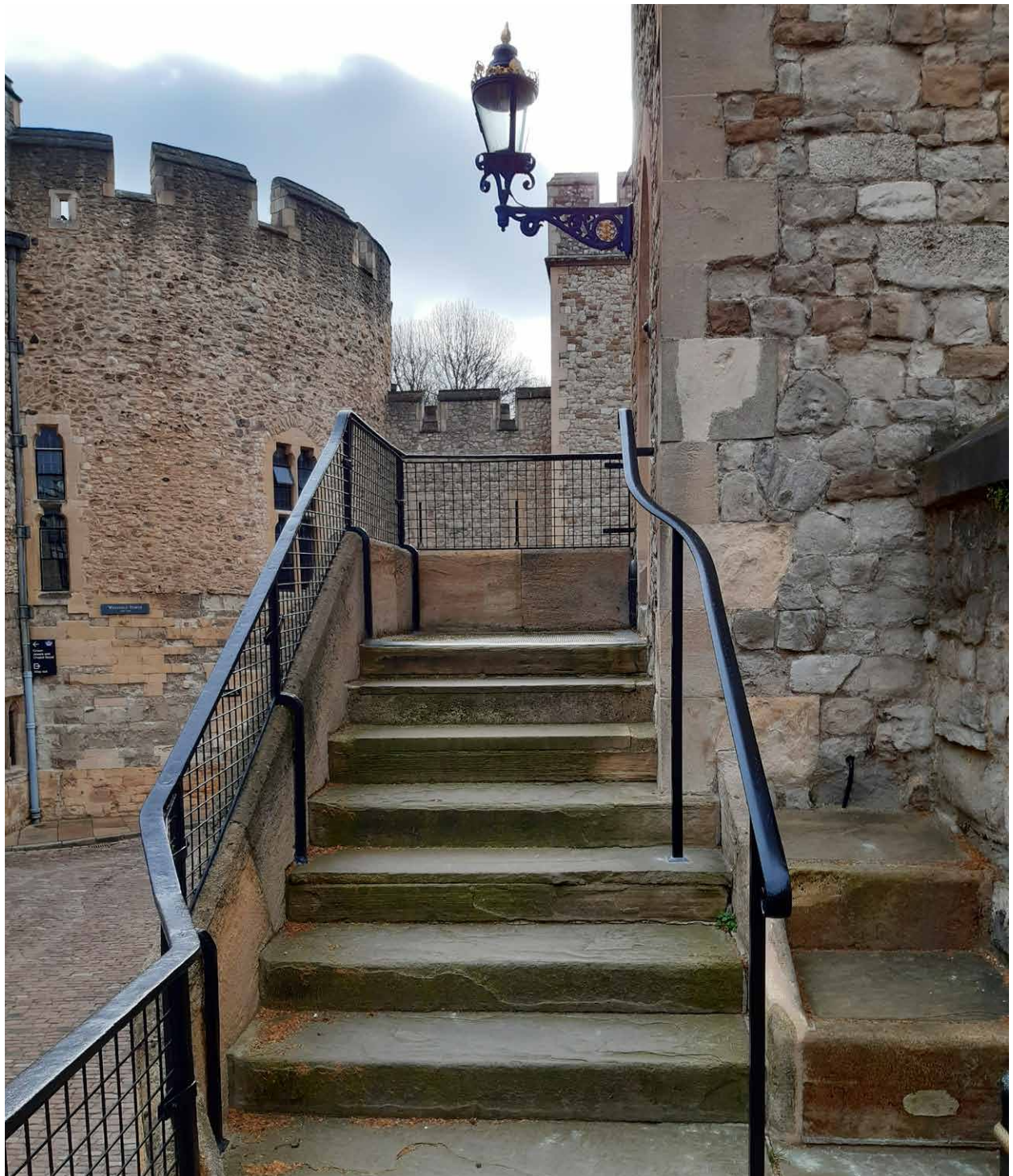
New wrought-iron handrails outside St Thomas' Tower, Tower of London, made by Stearn Metalworks to a design by Andrew Harris of Martin Ashley Architects and installed by Hall Conservation. The project was grant-funded by the Government's Culture Recovery Fund. © Historic Royal Palaces
