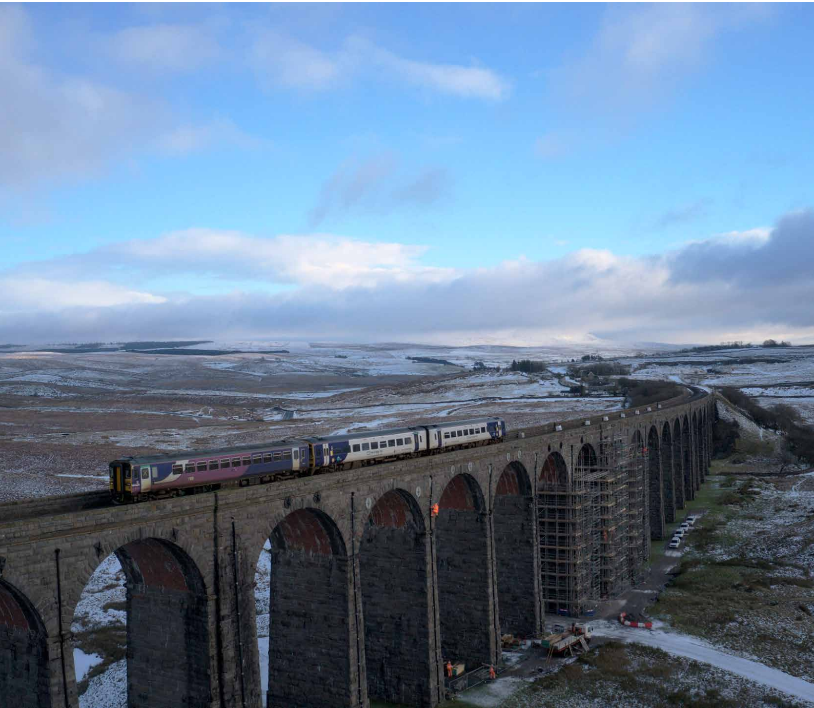
The Grade II*-listed Ribbleshead Viaduct being repaired in 2020-21, securing its future as both an historic landmark and vital railway link on the Settle-Carlisle railway line. © Network Rail
