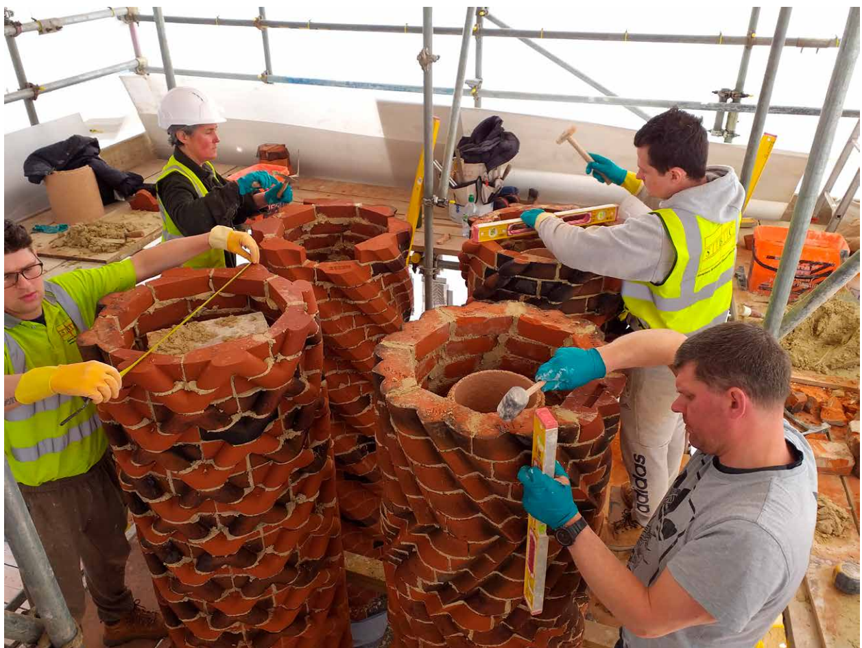
Simpson Brickwork Conservation at work rebuilding the chimney stacks to Apartment 23 at Hampton Court Palace, dismantled previously due to health and safety concerns. The project was grant-funded by the Government's Culture Recovery Fund. © Historic Royal Palaces
