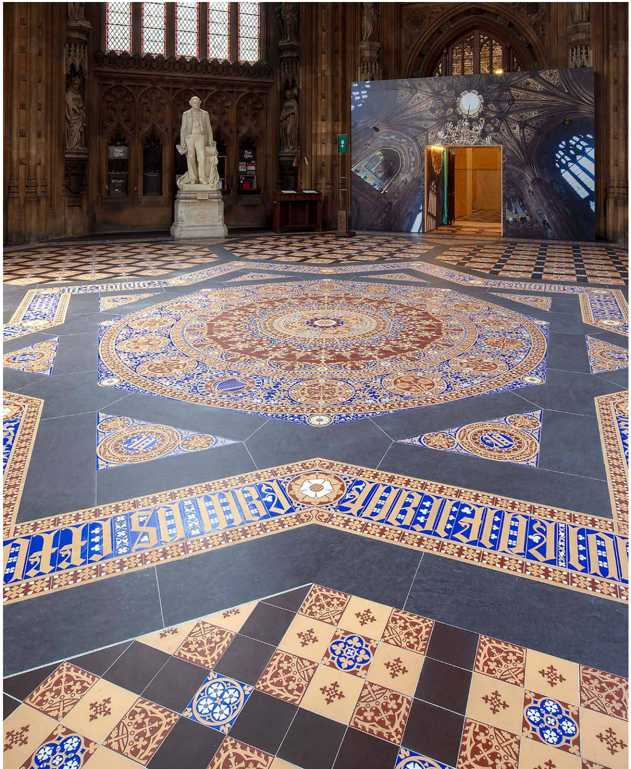
Encaustic tile and slate pavement, Central Lobby, following conservation. © UK Parliament / Adam Watrobski
