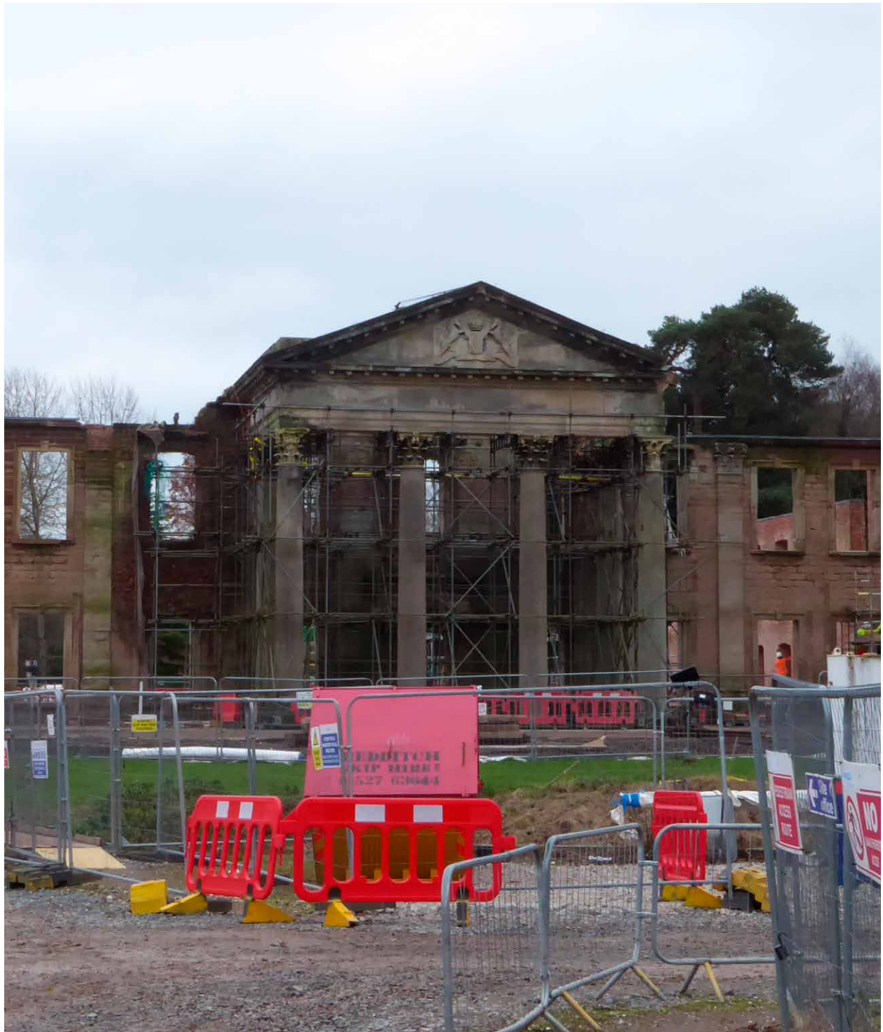
Major repair works are in progress to the Grade II-listed ruins of the old Hewell Grange. Most of the structure is now stabilised and repaired and a final phase of works due to commence in 2022. The site is now on the market as the Ministry of Justice seeks to dispose of it.
