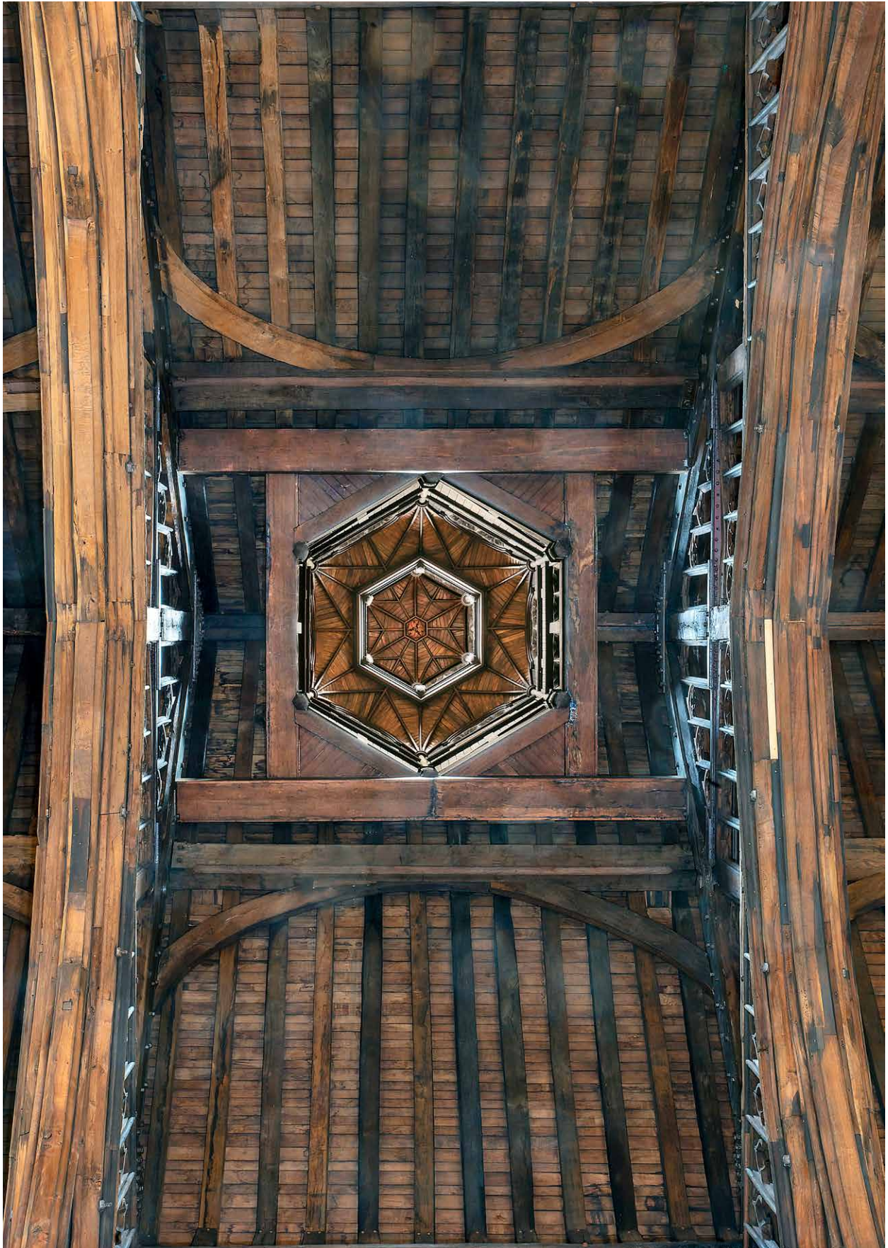
Interior of the renovated lantern on the roof of Westminster Hall, from below. © UK Parliament / Adam Watrobski
