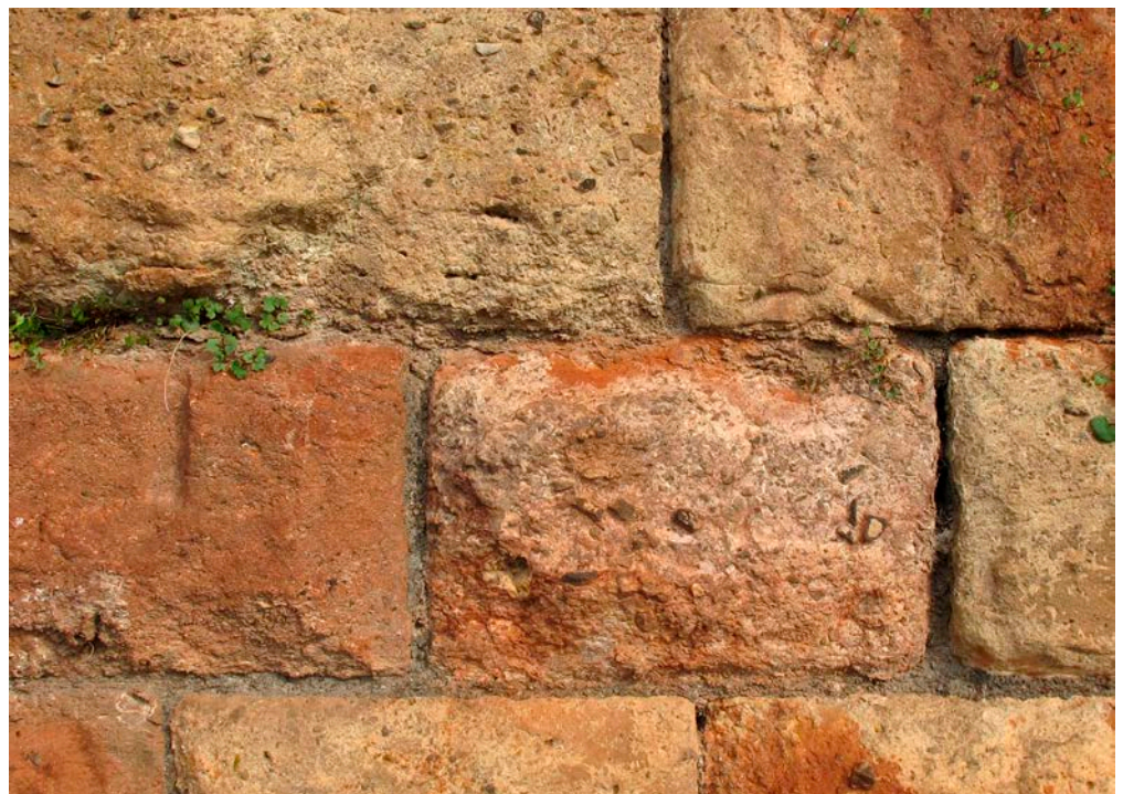
Figure 14: Walling, College Road, Clifton, Bristol. Deep red Dolomitic Conglomerate used with Carboniferous Limestone and Oolitic Limestone.
