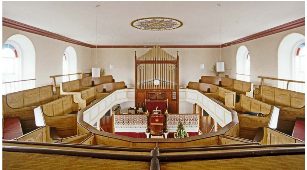
Figure 38: Gallery pews with grained decoration in the 1860 Wesleyan Reform Union chapel at St Just (Grade II). The photograph also shows the fine ceiling rose, and looks towards the organ loft set above the rostrum. This dates from 1895, and incorporates part of the original bow-fronted pulpit. The organ is possibly later. © Eric Berry
