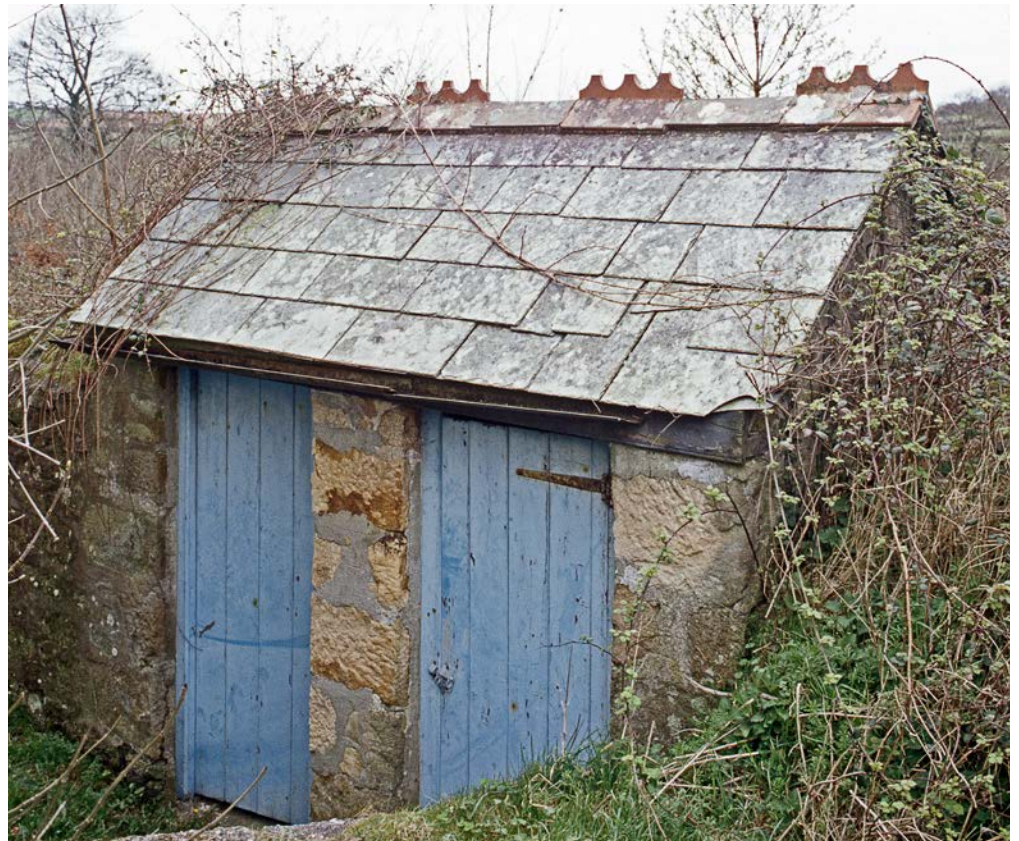
Figure 47: Small-scale ancillary buildings such as these earth closets at Coombe, St Stephen in Brannel, are rare. © Eric Berry
