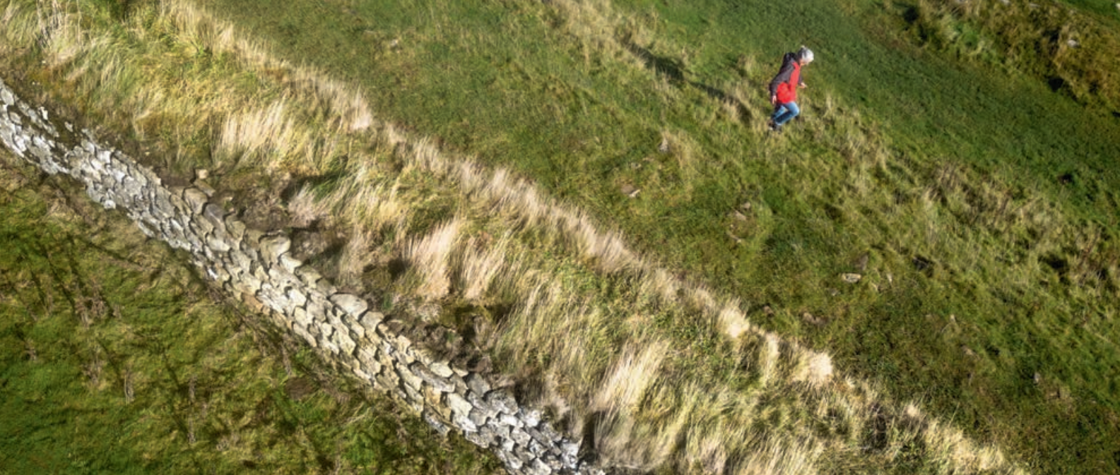
Steel Rigg, Hadrian's Wall, Northumberland. With a Heritage at Risk grant, soft capping was added to this section of wall to keep people from walking along the top of the wall causing damage and collapse
