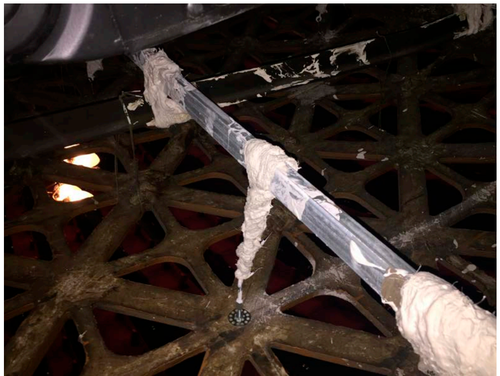
Figure 33: Fibrous plaster fretwork, given supplementary support with a new beam and wire-reinforced wads. This is a standard method of improving the stability of suspended ceilings.
