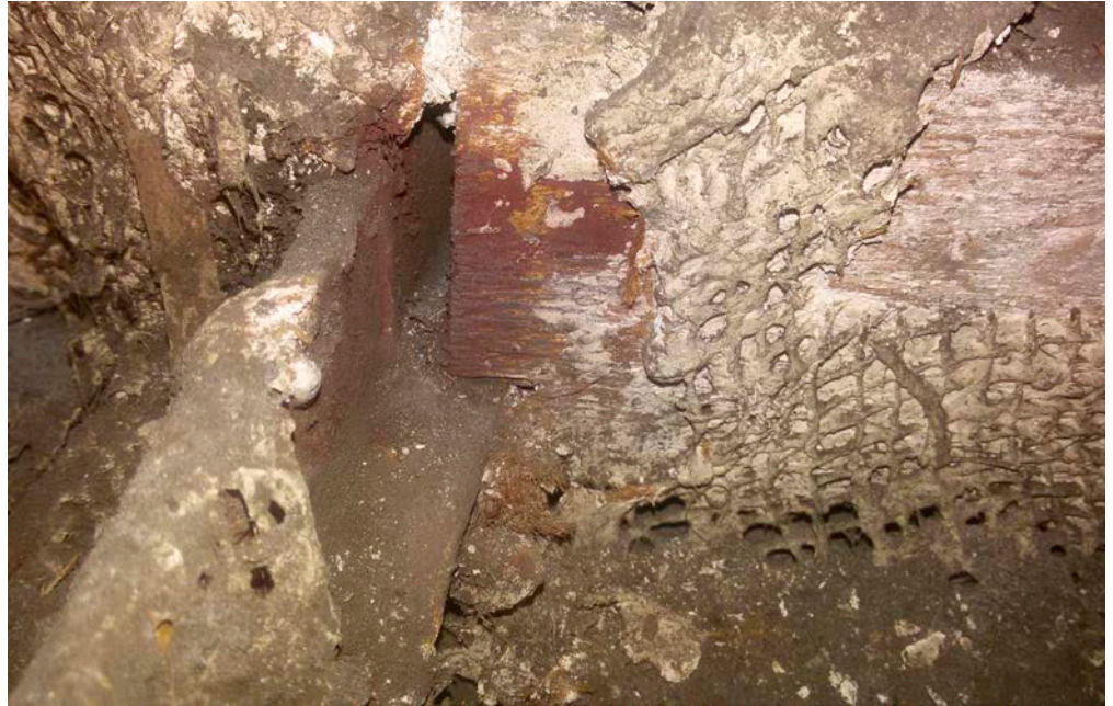
Figure 30: Poor bearing of a timber ceiling joist on a small steel T bar. The hessian has insufficient plaster cover to protect it from degradation. This illustrates how defects can be concentrated.
