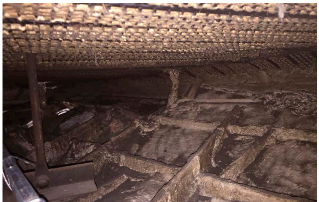
Figure 29: Large area of ceiling installed without sufficient wad connections to the panels. This can be easily detected in an inspection and remedied in subsequent repairs.
