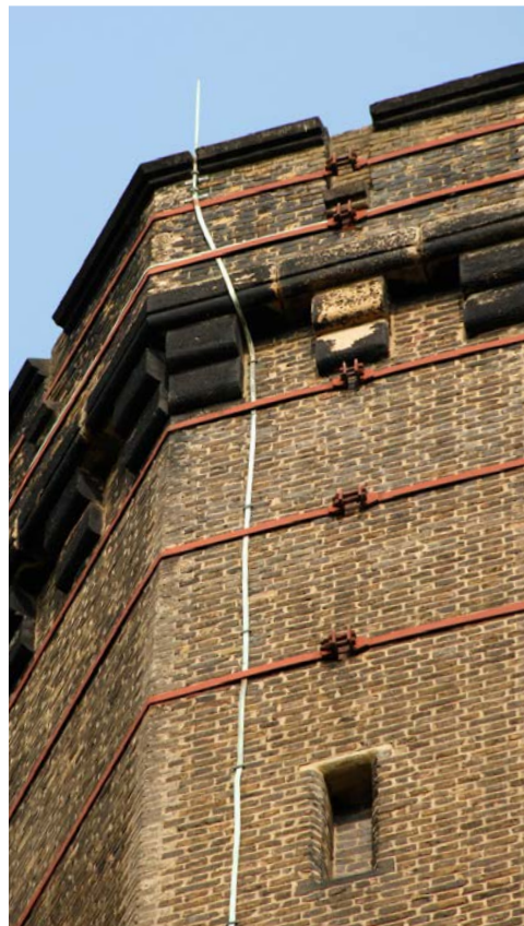
Figures 7, 8: Examples of lightning conductors on a water tower and a chimney.
