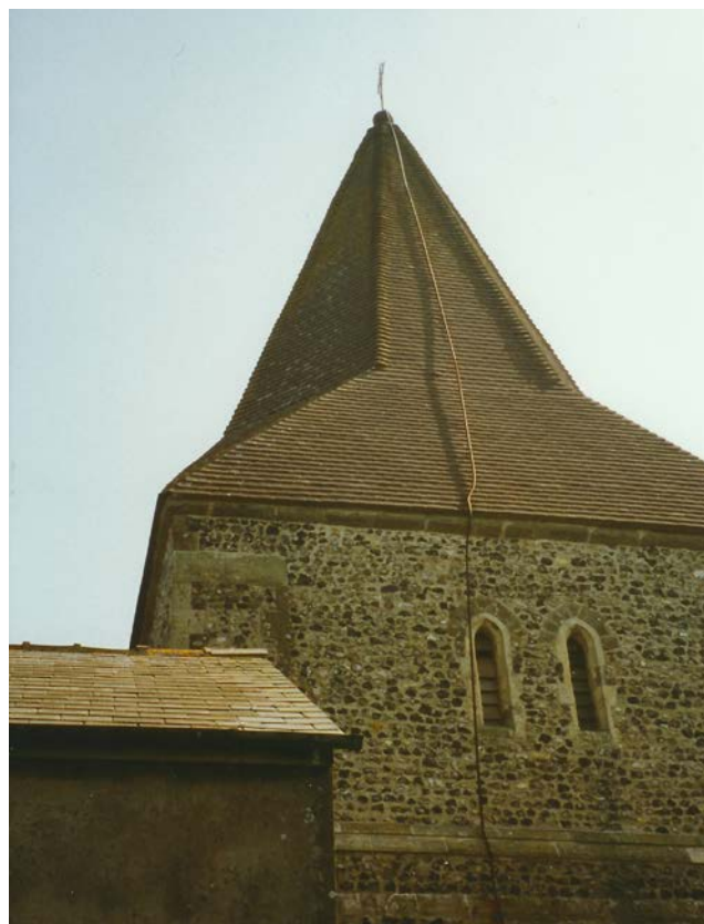
Figure 16: A very old and unusual iron conductor made of screwed sections at St Lawrence's Church, Hougham (Kent). Note the lack of support of the roof section.
