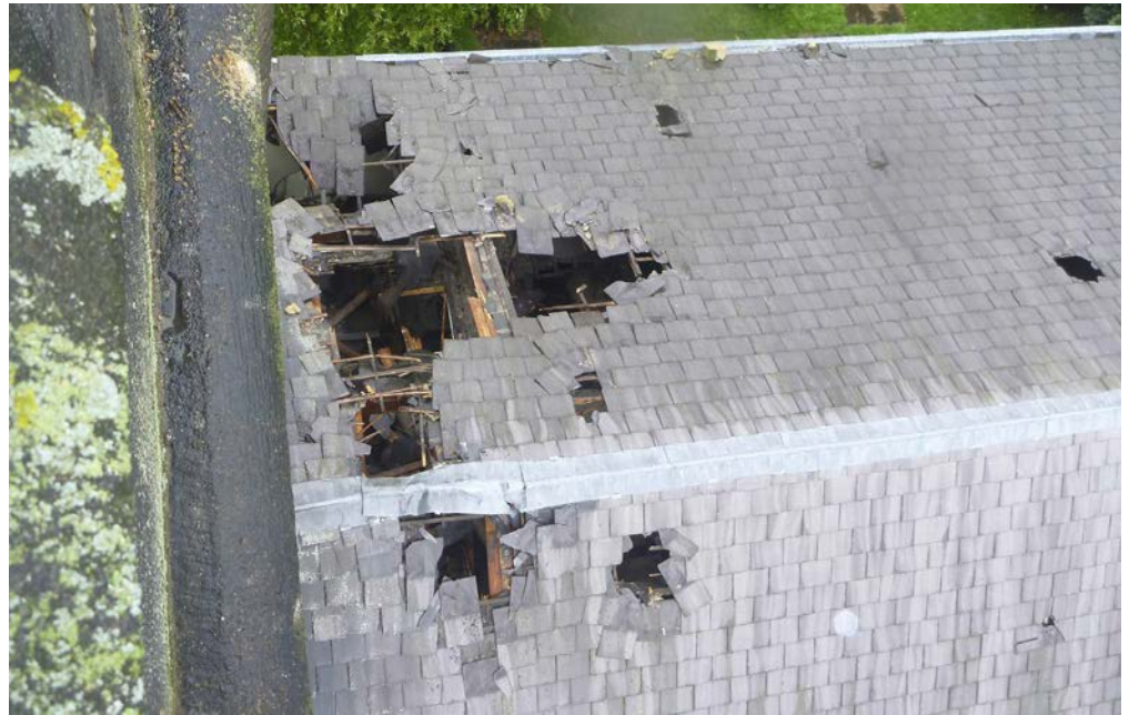
Figure 3, 4: Masonry debris from the tower fell through the roof of St Andrew's Church, Ramsbottom (Bury) causing extensive damage.
