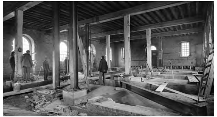
Fig. 306. J057/03/72. (28 Apr 1971). Photograph of Storehouse No. 11, ground floor conversion to the McCarthy Museum. ©Crown copyright.HE.
