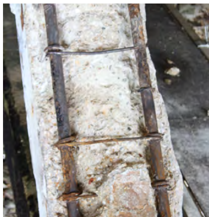
Fig. 236. Underside of a Portsmouth Boathouse No. 4 (1940, 1/6) concrete truss, showing its corroded iron reinforcing bar. A. Coats 2015. Reproduced with the kind permission of Portsmouth Naval Base Property Trust.
