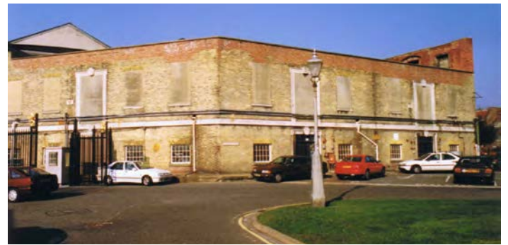
Right: Fig. 266. Portsmouth Boathouse No. 6. Photograph of the east end, south and east elevations, showing the missing roof after the air raid. PNBPT Record Photograph no. E07 (June 1998). Reproduced with the kind permission of Portsmouth Naval Base Property Trust.
