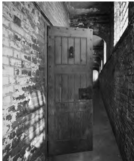
Fig. 215. J473/07/71. Photograph of the Cell Block Interior: first floor cell door (8 Oct 1971). ©Crown copyright. HE.
