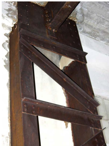
Fig. 244. Interior steel frame and beam of Portsmouth Boathouse No. 4 (1940, 1/6). A. Coats 2015. Reproduced with the kind permission of Portsmouth Naval Base Property Trust.
