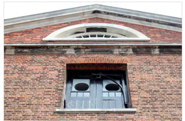
Fig. 316. A refurbished rear pediment of Portsmouth Storehouse No. 10 (1776, 1/59), showing the access doors to the upper floor and cast iron bracket (2014). A. Coats 2014. Reproduced by kind permission of the Trustees of the National Museum of the Royal Navy.
