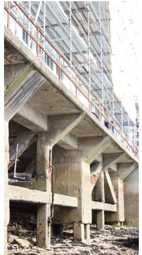
Fig. 232. West elevation of the undercroft of Portsmouth Boathouse No. 4 (1940, 1/6) at low tide, showing its beams and trusses. A. Coats 2015. Reproduced with the kind permission of Portsmouth Naval Base Property Trust.
