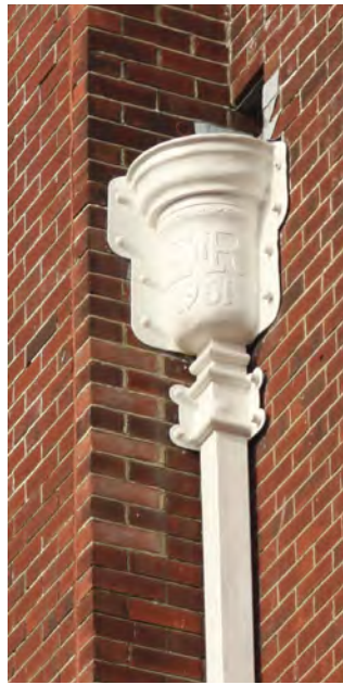
Fig. 328. Rainwater hopper dated 1961, west elevation of Portsmouth Fleet Headquarters, Jago Road (1961, 1/80). A. Coats 2014. Reproduced with the permission of the MoD.
