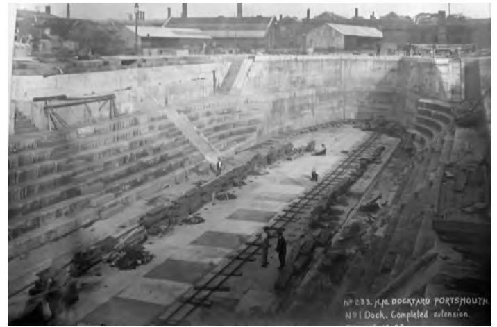
Fig. 335. Dock No. 1 (6.1.1909). Photograph of completed extension, looking northeast. TNA, ADM 195/79 (1857–1915). 100 photographs depicting construction works at Portsmouth Dockyard. Reproduced with the permission of The National Archives.
