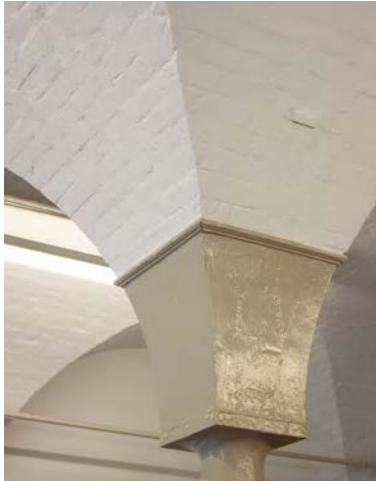
Fig. 255. Interior of Portsmouth Pay Office (1808, 1/11), showing the cast iron bases to the vaulted brick ceiling columns. A. Coats 2012. Reproduced with the kind permission of Portsmouth Naval Base Property Trust.
