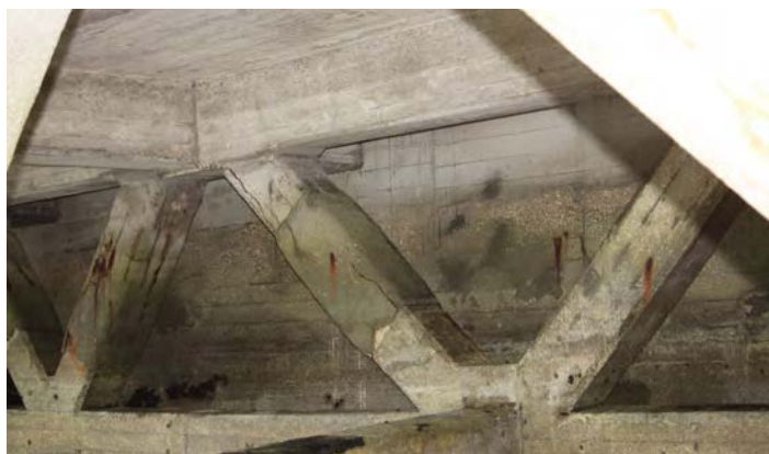
Fig. 233. Northern extent of the concrete and steel trusses forming the undercroft of Portsmouth Boathouse No. 4 (1940, 1/6) on its west (harbour) elevation, showing the shuttered concrete west seawall. A. Coats 2015. Reproduced with the kind permission of Portsmouth Naval Base Property Trust.
