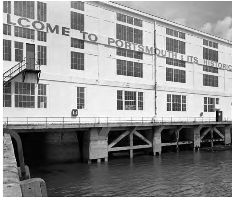
Fig. 229. BB97/09274. West elevation of Boathouse No. 4 showing the concrete supporting trusses at high tide (28 Jul 1997). ©Crown copyright.HE.
