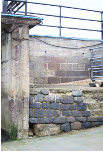
Fig. 239. Southern extremity of the seawall of Portsmouth Boathouse No. 4 (1940, 1/6), sitting on the older and only operational patent slip in the naval base. A. Coats 2015. Reproduced with the kind permission of Portsmouth Naval Base Property Trust.
