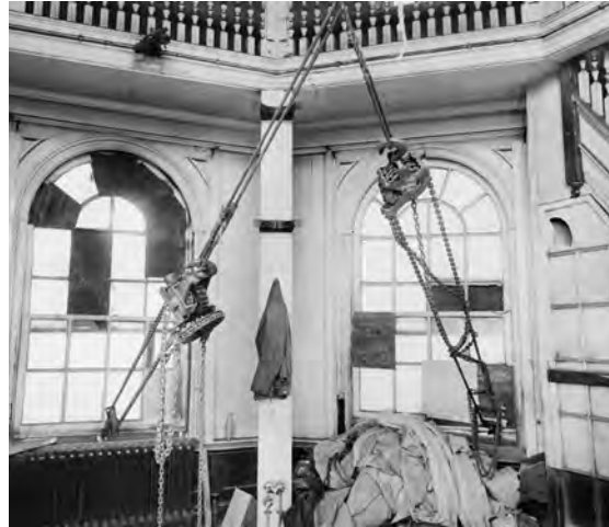
Fig. 256. P241/53 FL00981/01/001. Photograph showing progress of the reconstruction of the Former Naval Academy's cupola, following its bomb damage in 1941 (09 Mar 1953). Reproduced by permission of Historic England.
