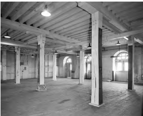
Fig. 309. J186/06/71. Photograph of Storehouse No. 9, 10 or 11 (28 Apr 1971). ©Crown copyright.HE. It is hoped that the particular storehouse can be identified.
