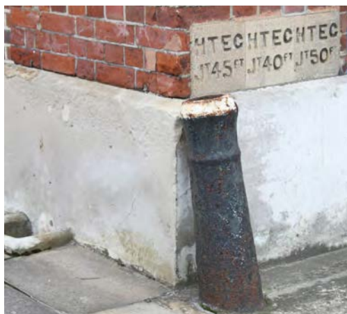
Fig. 353. Cannon protecting the northeast corner of the former Portsmouth Chief Inspector's Office (1857, 1/138). A. Coats 2013. Reproduced with the permission of the MoD.
