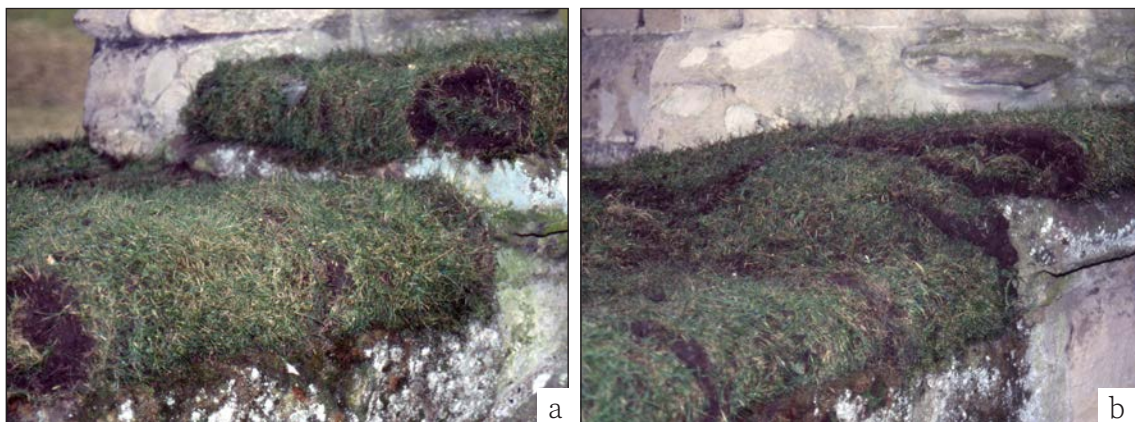
Figure 6.5 (a) soft capping above and below the step initially retains its appearance (right hand side), but this will be lost to some extent as the grass grows, (b) ramping over the step means a loss of definition but increased fabric protection. (both ©Alan Cathersides)
