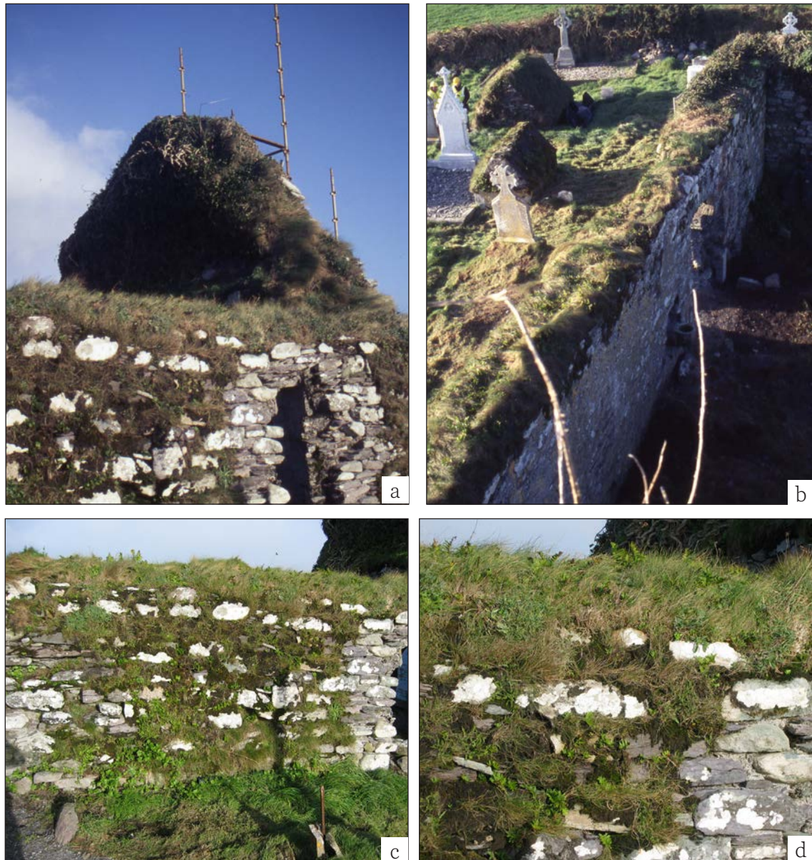
Figure 1.5 (a-d) Natural soft capping at Myross Church, County Cork, Ireland. (a-b © Alan Cathersides, c-d Chris Wood ©Historic England)
