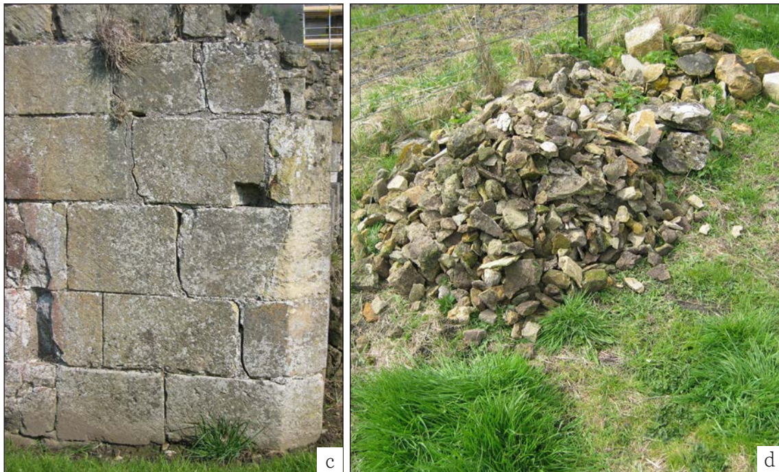
Figure 2.2 Deterioration at Byland Abbey
