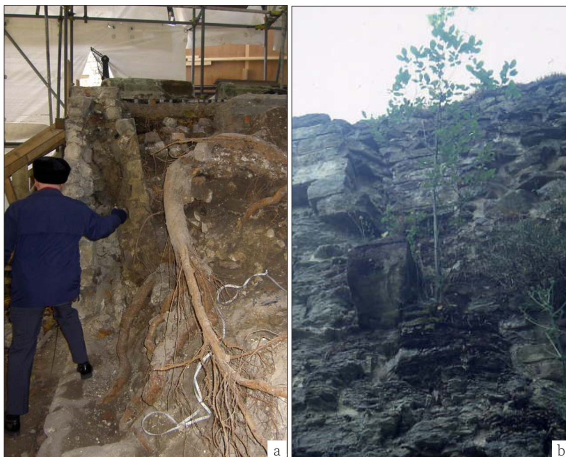
Figure 6.11 Damage to the moat wall at the Tower of London (a) caused by the secondary thickening of tree roots; and a tree growing on an uncapped ledge on a wall at Wigmore Castle (b). (both ©Alan Cathersides)
