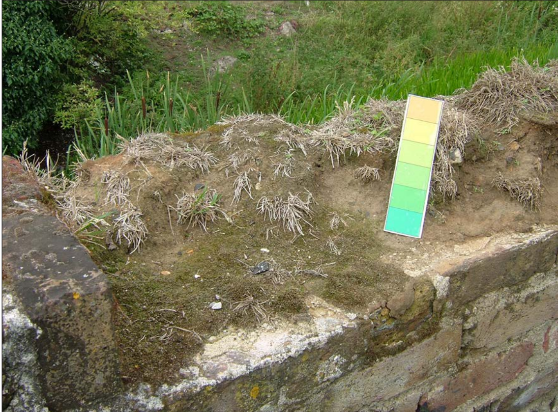
Figure 4.35 Failed soft capping at Howbury moated site (Photo taken in 2010). ©Heather Viles, University of Oxford
