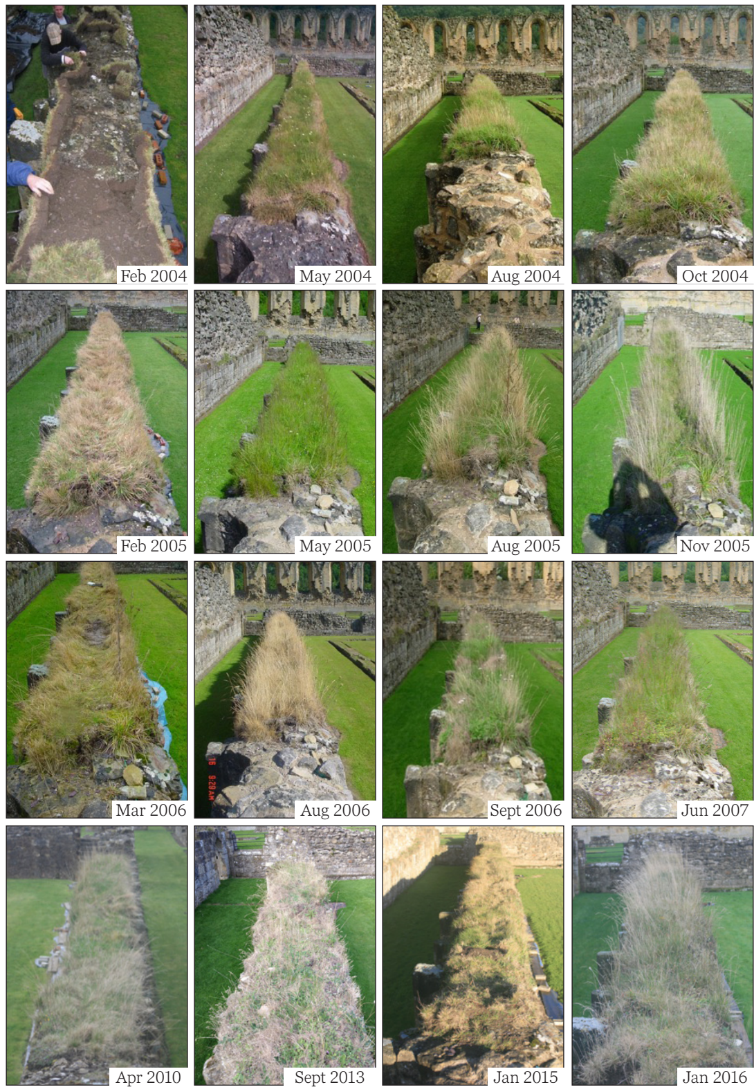
Figure 4.31 Byland Abbey soft capping on the Lane wall (Feb 2004–Jan 2016). ©Heather Viles, University of Oxford
