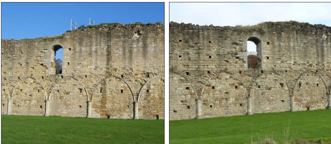
Figure 4.28 Streaking at Kirkham Priory in (a) 2014 and (b) 2016.
