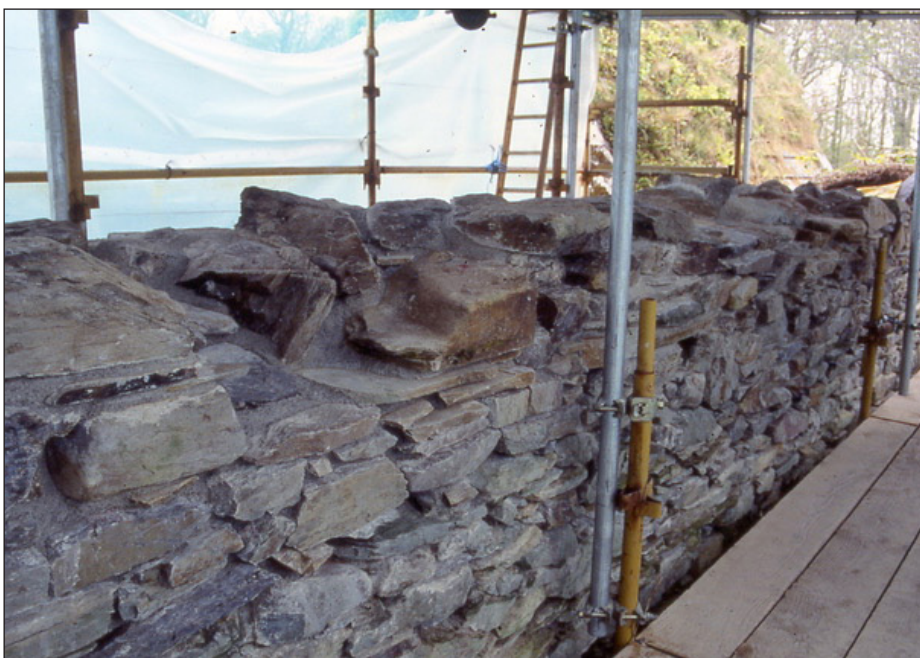
Figure 6.16 (top) (a) Cleaning the surface to prepare it for rebuilding, and (b) starting to rebuild the wall in levels across the wall. Figure 6.17a,b (bottom) The wall near completion, showing good continuity with the rest of the structure. (all ©Colin Burns)
