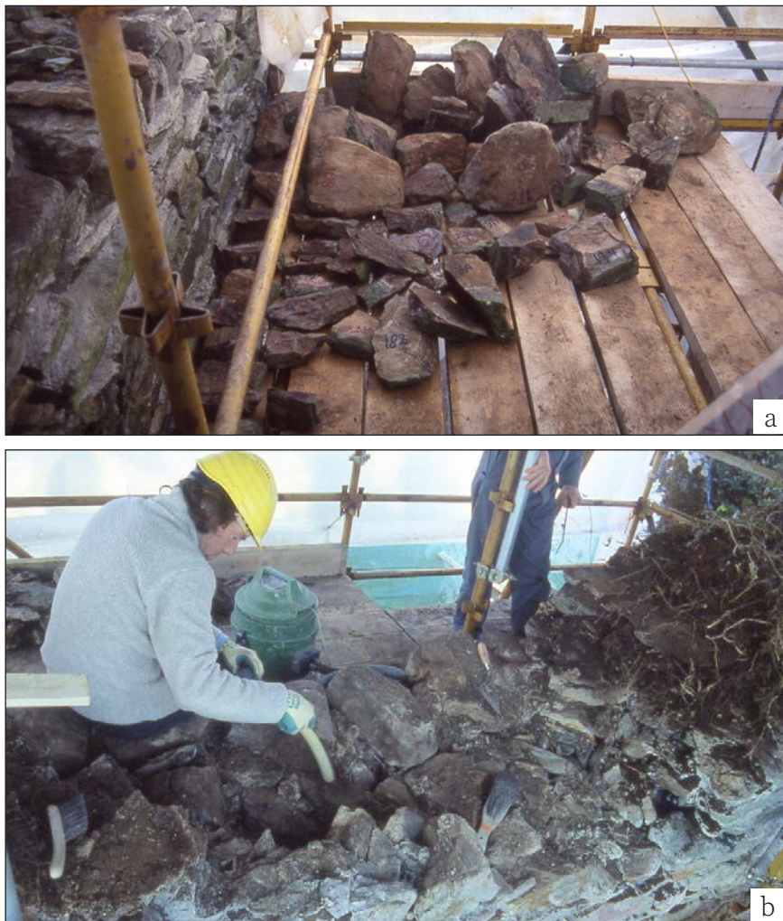
Figure 6.15 (a) Numbering and labelling the face work stones as they are removed from the wall, and (b) removal and cleaning of the core work. ©Colin Burns
