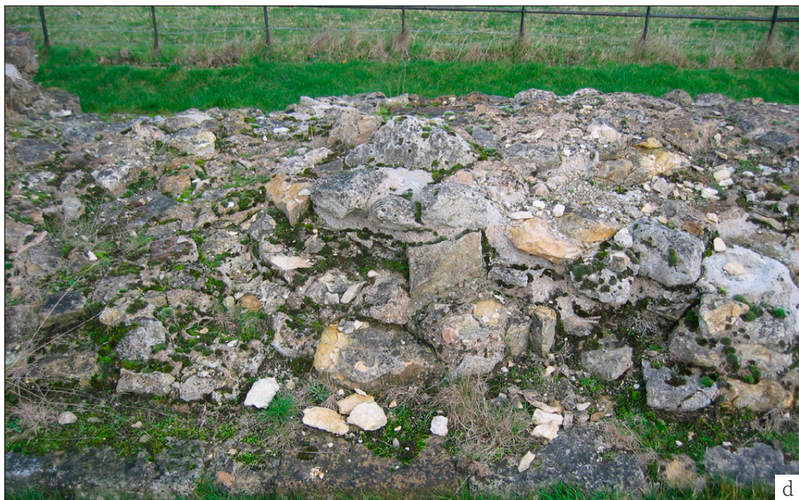
Figure 2.6 c,d Frost damage at Thornton Abbey on (a) brick and (b) stone. Image (a) shows a pile of frost-shattered brick debris swept carefully from the surrounding brick surface. (both ©Heather Viles, University of Oxford)
