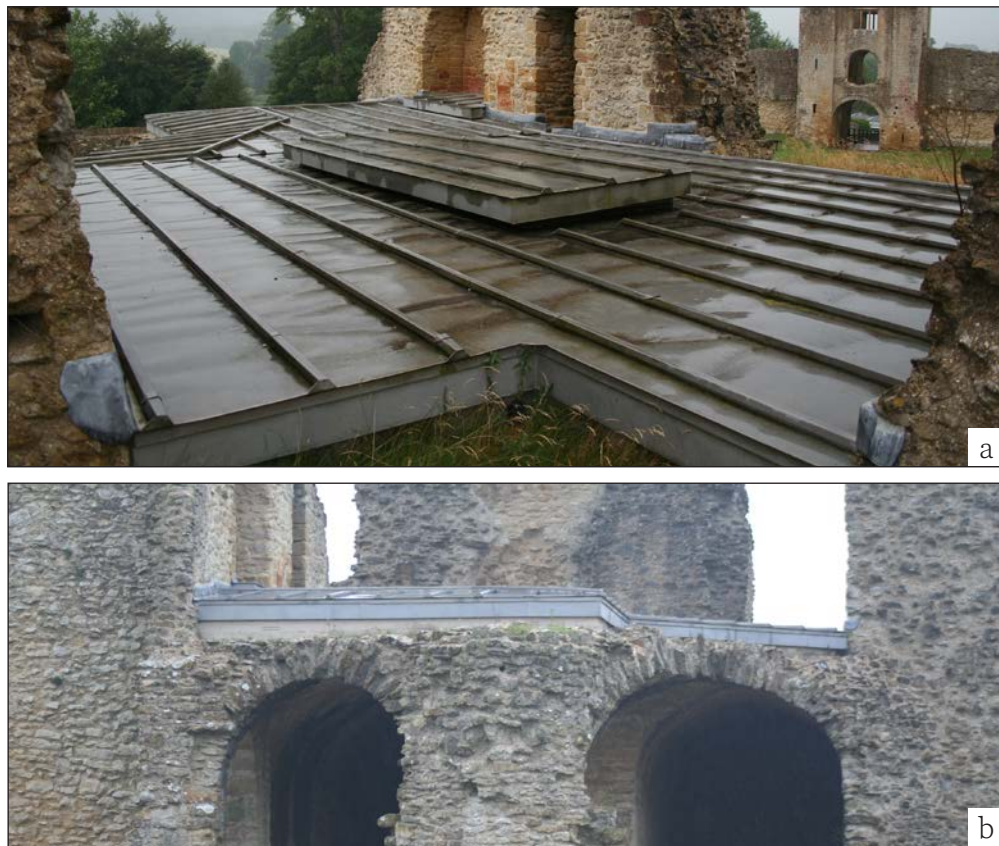
Figure 7.9 A flat zinc roof built at Sherborne Old Castle to tackle problems of water ingress. (both ©Chris Wood, Historic England)
