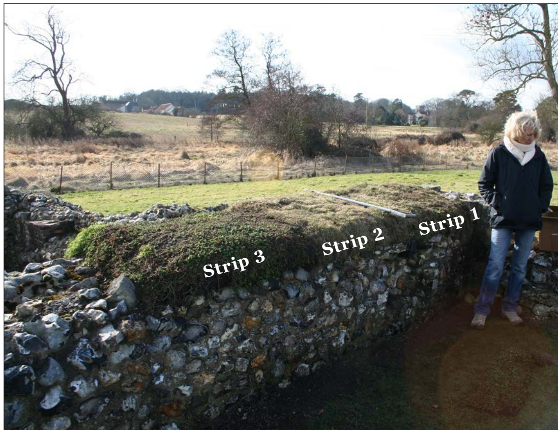
Figure 2.17 Soft wall caps installed at Castle Acre Priory, February 2012. ©Heather Viles, University of Oxford
