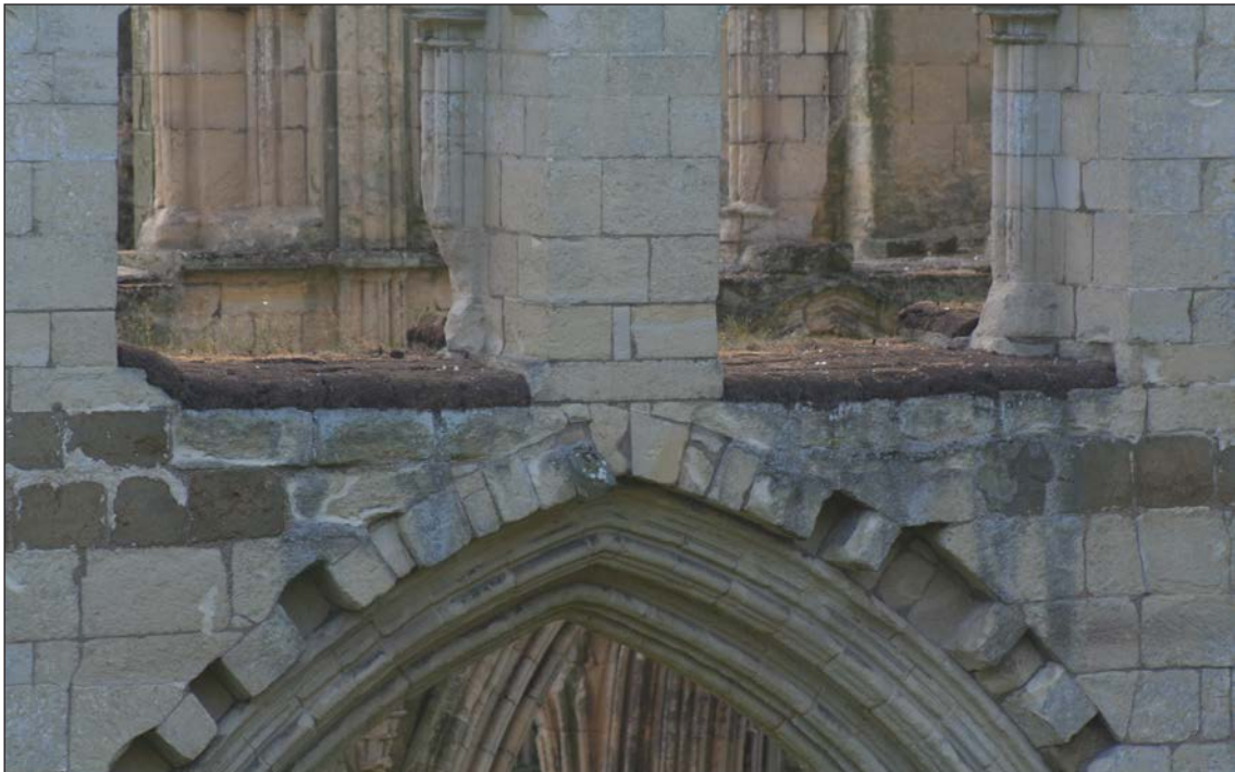
Figure 4.36 Failed soft capping at Rievaulx Abbey. ©Heather Viles, University of Oxford
