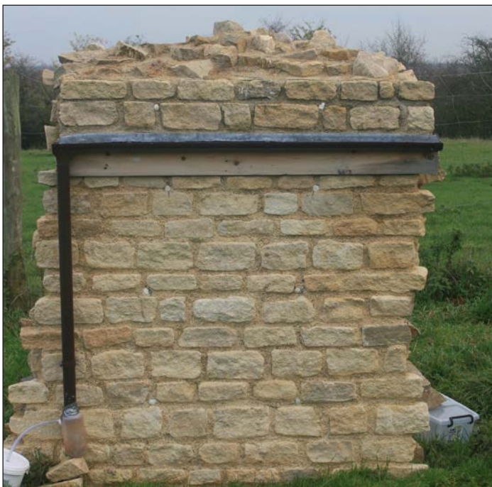
Figure 3.15 Guttering with lead flashing to collect runoff. ©Heather Viles, University of Oxford
