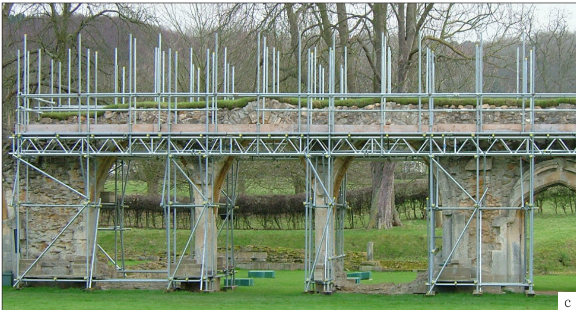
Figure 2.12c Soft capping was installed over the wall head in the east cloister at Hailes Abbey, where previous consolidation and lime mortar repairs had been carried out. ©Heather Viles, University of Oxford
