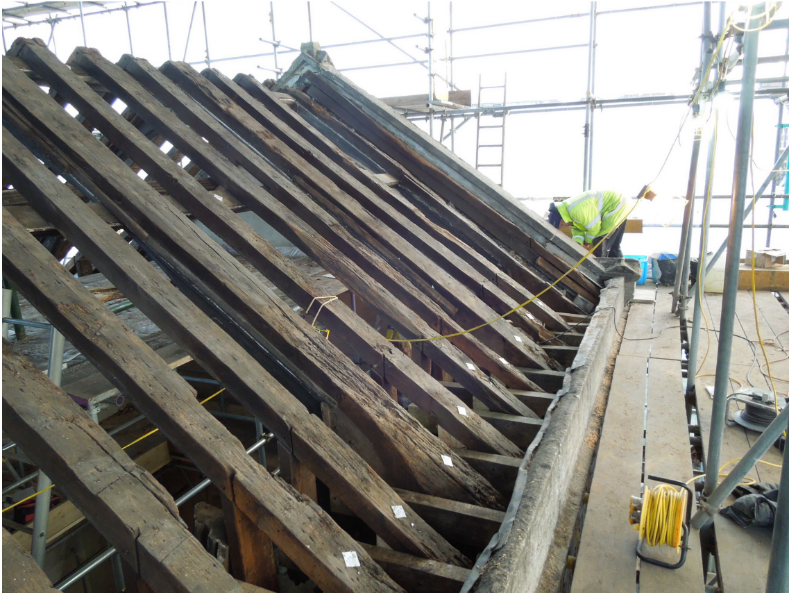
Figure 2: View of the south slope of the chancel roof (looking east), showing the exposed rafters (photograph Martin Bridge)
